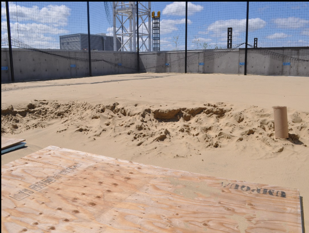
Beach sand at rooftop volleyball court
